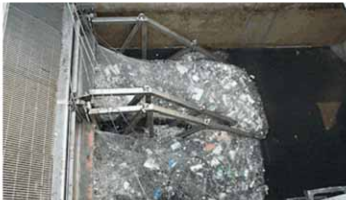
End of pipe netting on a North Bergen, NJ, CSO ready to be changed out
