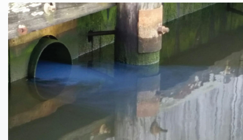
Abnormal blue, shiny discharge from an overflow stormwater drain
